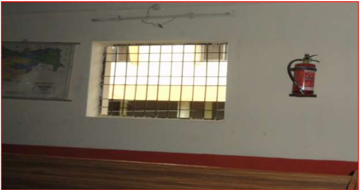
Fire Extinguisher available in the library
